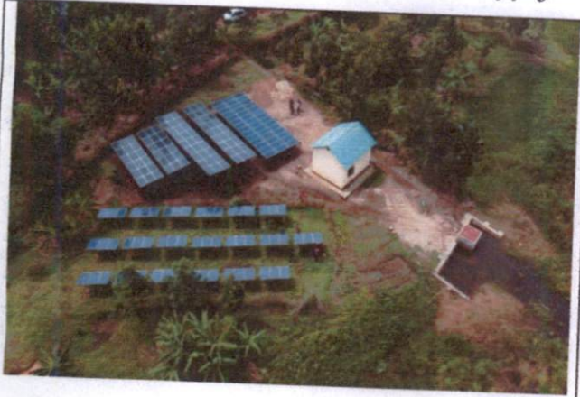
Solar panels for irrigation system
