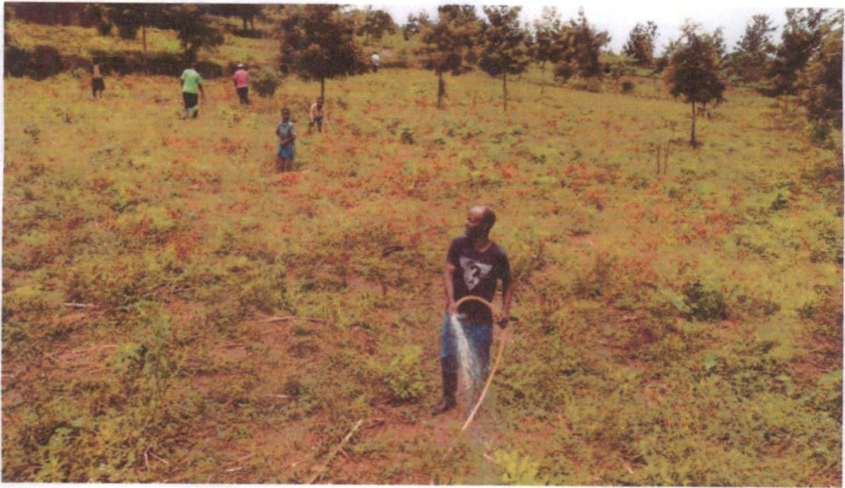
Solar irrigation system installed in the buffer zone of Murago wetland
