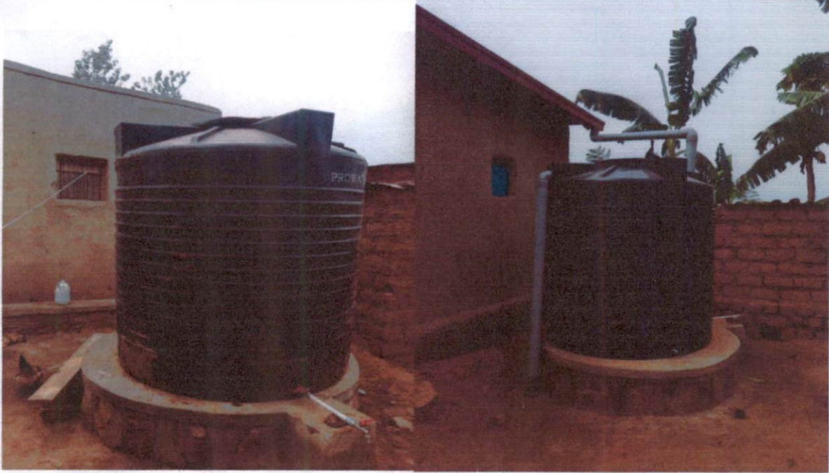
Installed water tanks in 254 households of Rugarama cell, Mareba Sector
