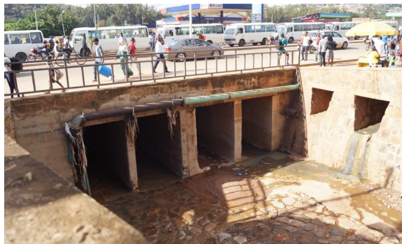
FIGURE 11. NYABUGOGO TRANSPORT HUB BRIDGE ON MPAZI CHANNELIZED RIVER THAT IS PERIODICALLY DAMAGED BY FLUSH FLOODING
