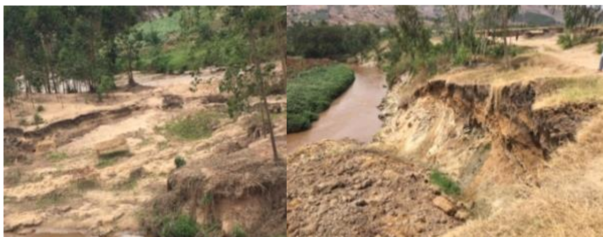
Figure 30. Gullies along the sloped banks of the Muvumba River as a result of intense rainfall runoff and soil erosion and low vegetation cover. Source: Theogene Habakubaho, September 2020.
